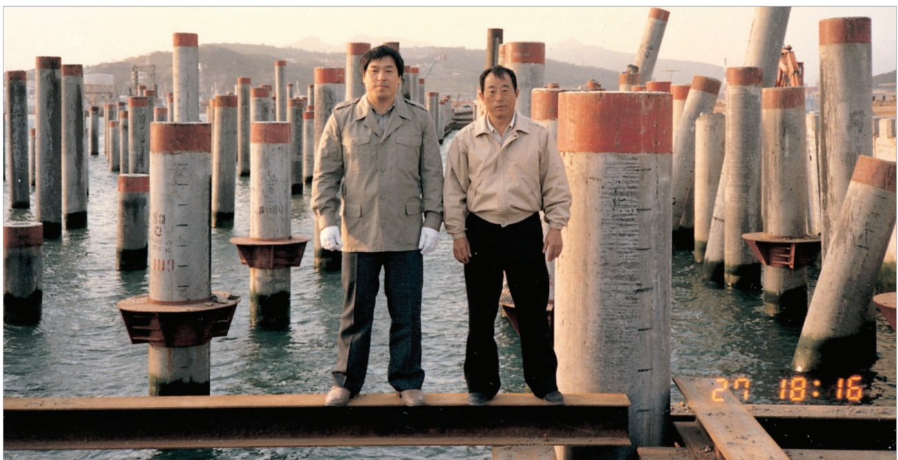
Chairman and CEO S. Joon Kim (left) visiting the pier-type quay wall construction site of the “Shinseondae” container port in Busan. The hundreds of piles on the sea symbolically demonstrate the complexity of the construction project (April 27, 1989)
